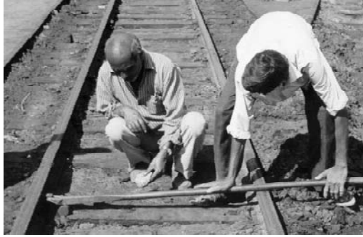
Figure 14 While using, crowbar touches the rail
